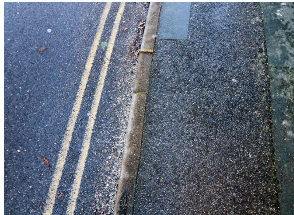
Figure 97: Unsympathetic tarmac pavements and concrete kerbs
