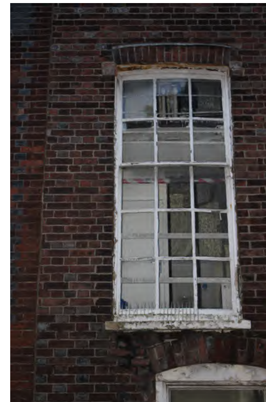
Figure 193: Pigeon spikes to the cill of a timber window in poor repair
