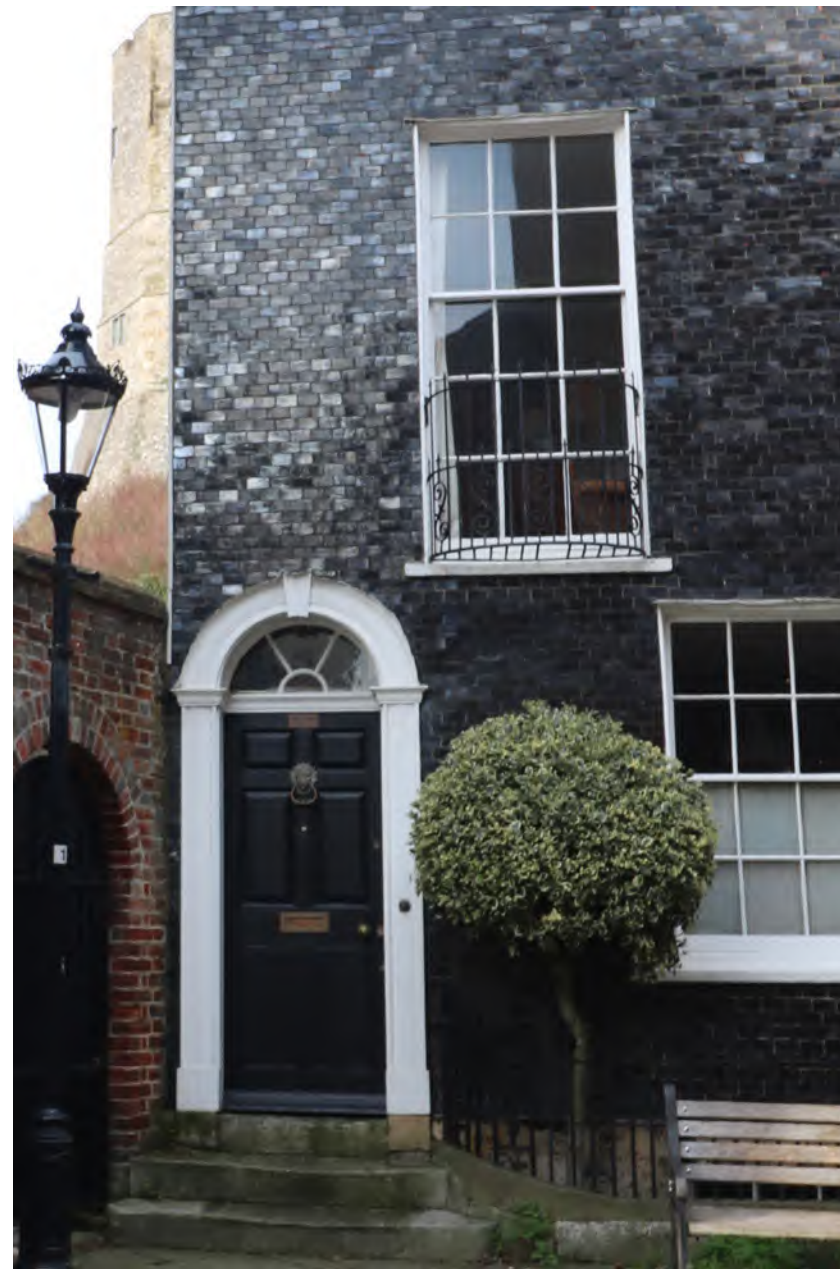
Figure 51: Vitrified mathematical tile to the façade of Bartholomew House. Note the lack of lintels over the openings
