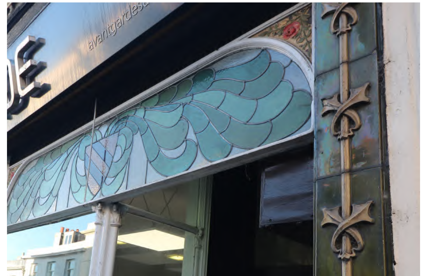
Figure 83: High Street shop front with slender transoms, a stained glass overlight and Late Victorian or Edwardian green glazed tiles to the edge of the shopfront
