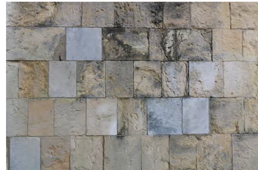
Figure 46: Close up of the Caen Stone to the façade of Dial House
