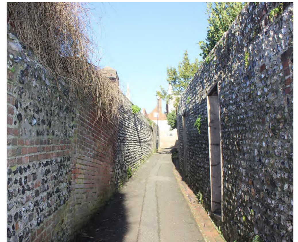
Figure 42: View along Paine's twitten. The flints protrude slightly beyond the surface of the pointing, creating a strong sense of texture
