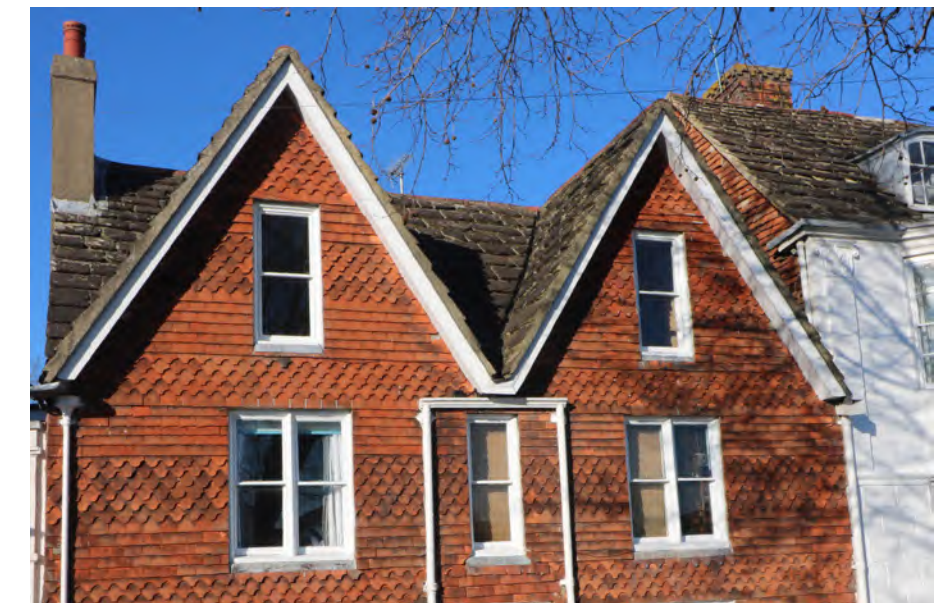
Figure 59: Horsham Stone slate roofs to Nos.55 and 56 Southover High Street. A steeper pitch is required than for slate
