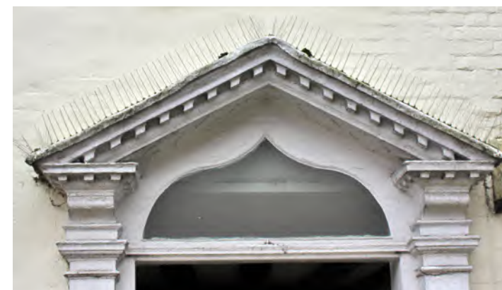
Figure 198: Pigeon spikes detracting visually from a characterful ogee door surround
