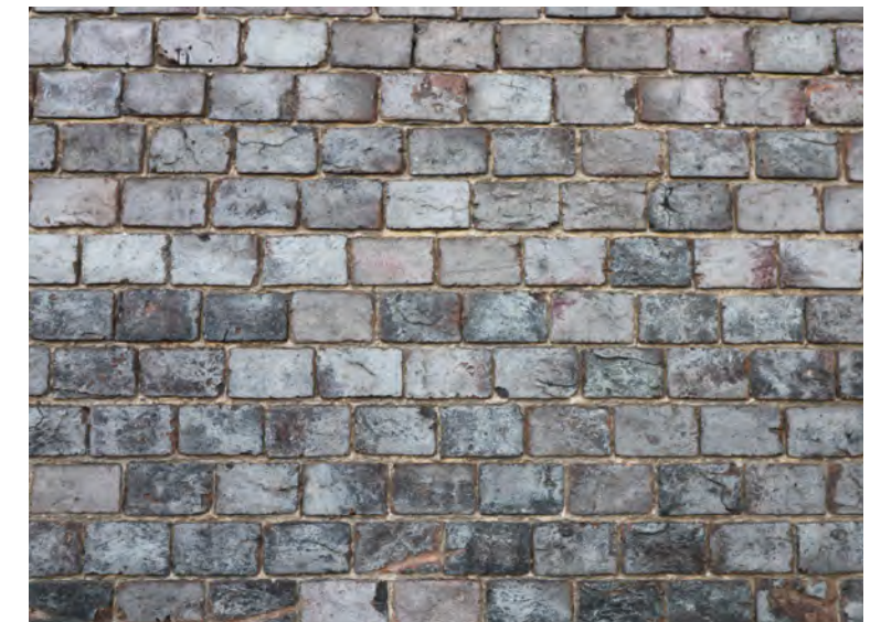
Figure 50: Grey brick headers. On close inspection the red undertones of the brick can be seen beneath the grey finish
