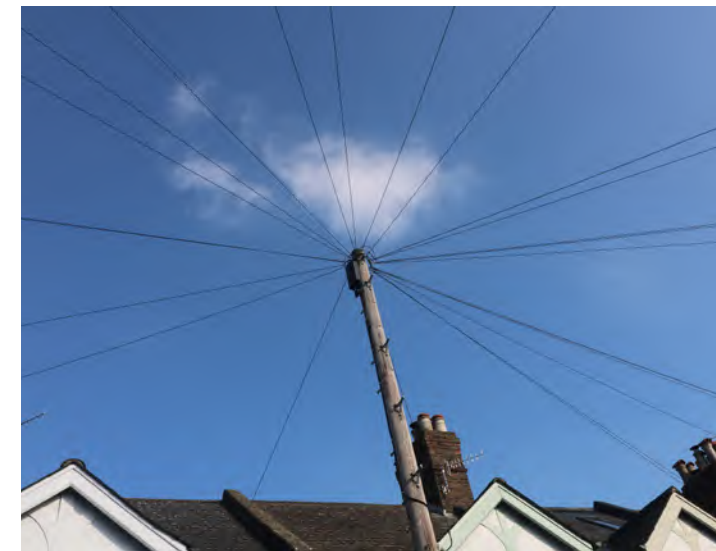
Figure 226: Visual clutter caused by power cables
