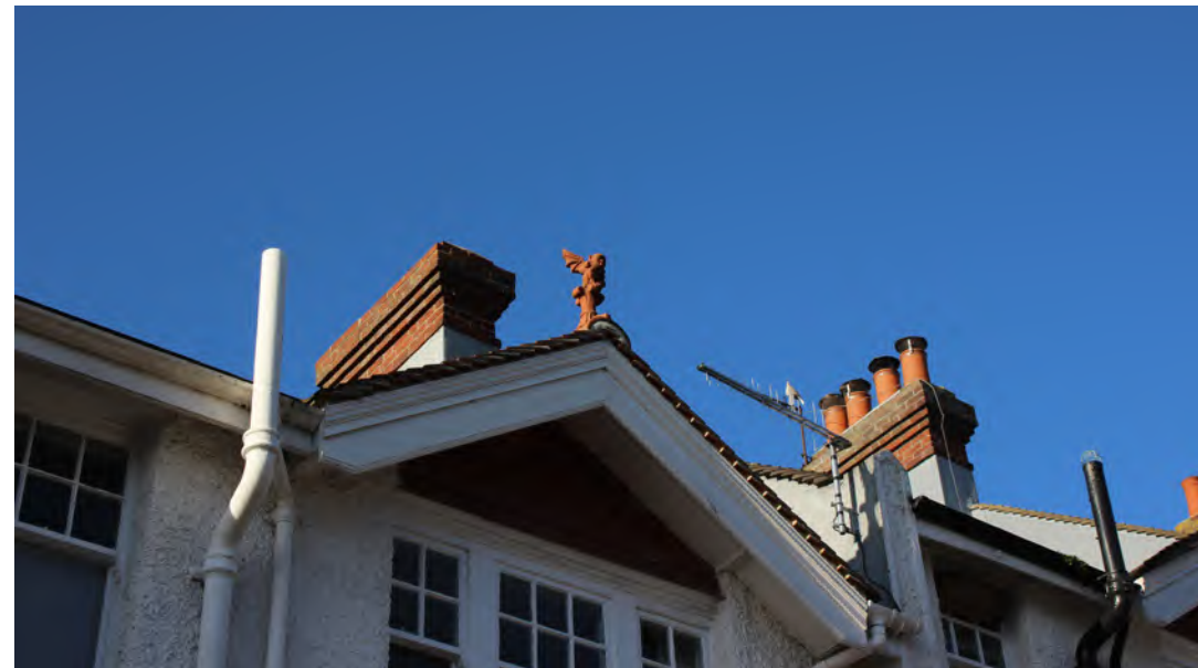
Figure 190: Cluttered drainage goods and TV antennae
