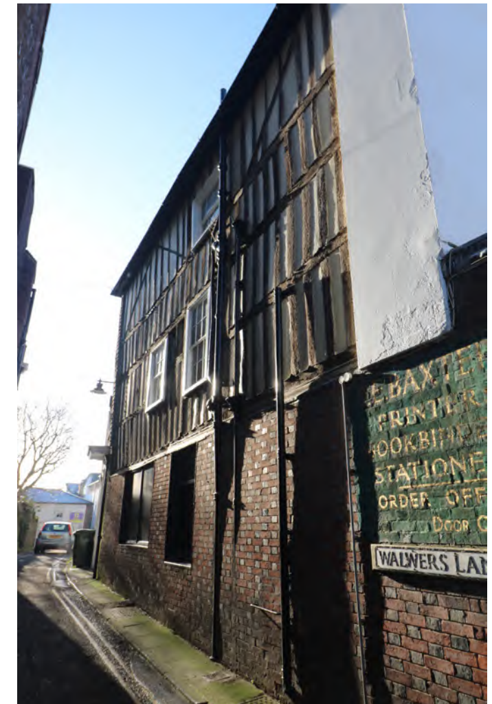
Figure 37: Relatively ornate timber framing to the gable end of the Arts and Crafts former Fruiterers Arms Pub on Sun Street.
