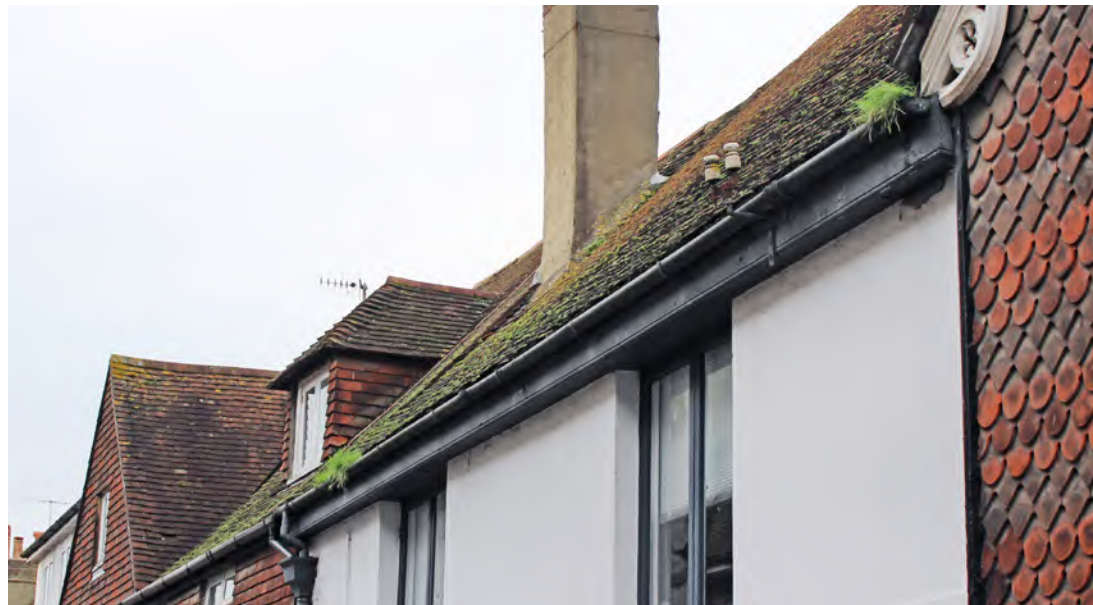
Figure 189: Vegetation growing in a blocked gutter on Cliffe High Street
