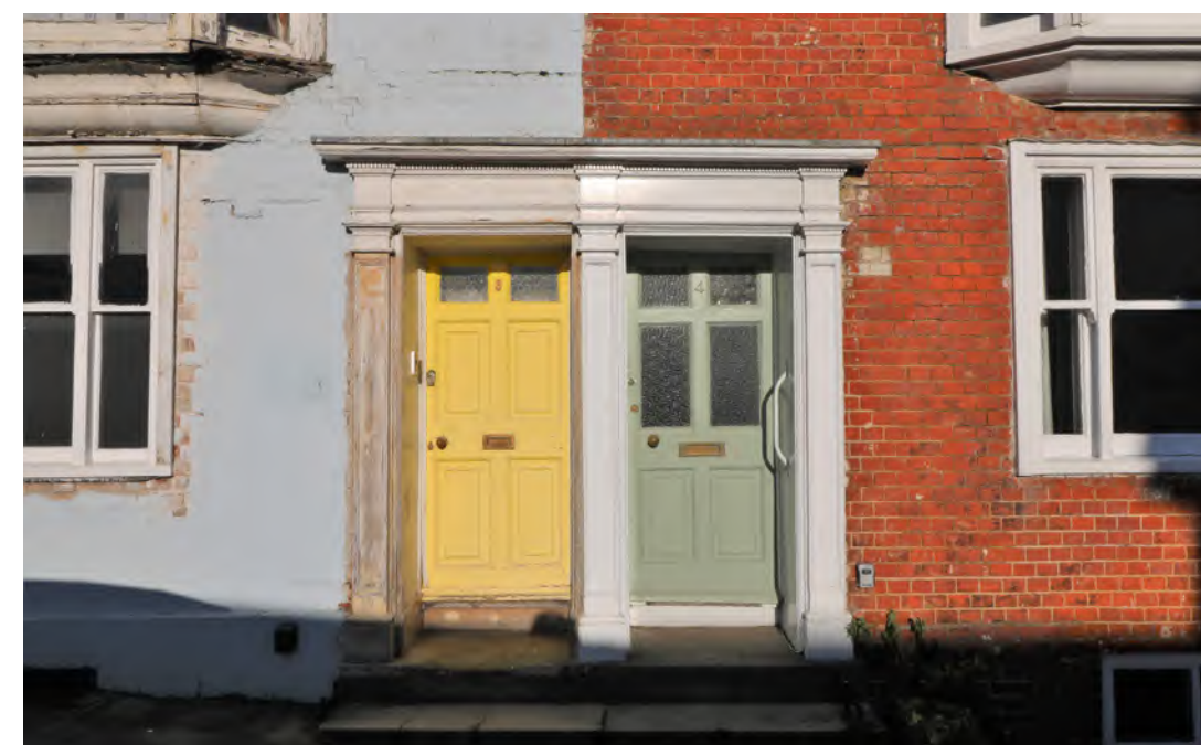
Figure 194: Neighbouring poorly-maintained and well-maintained houses, showing the impact of a lack of regular painting and maintenance on timberwork
