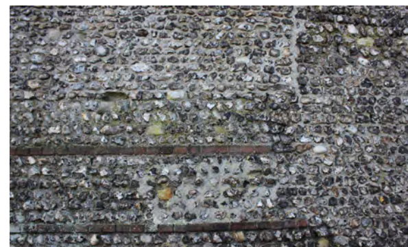
Figure 41: Flint boundary wall to Pelham House. The repair to the centre of the picture demonstrates the importance of consistency in pointing, the repair covering more of the flints in mortar
