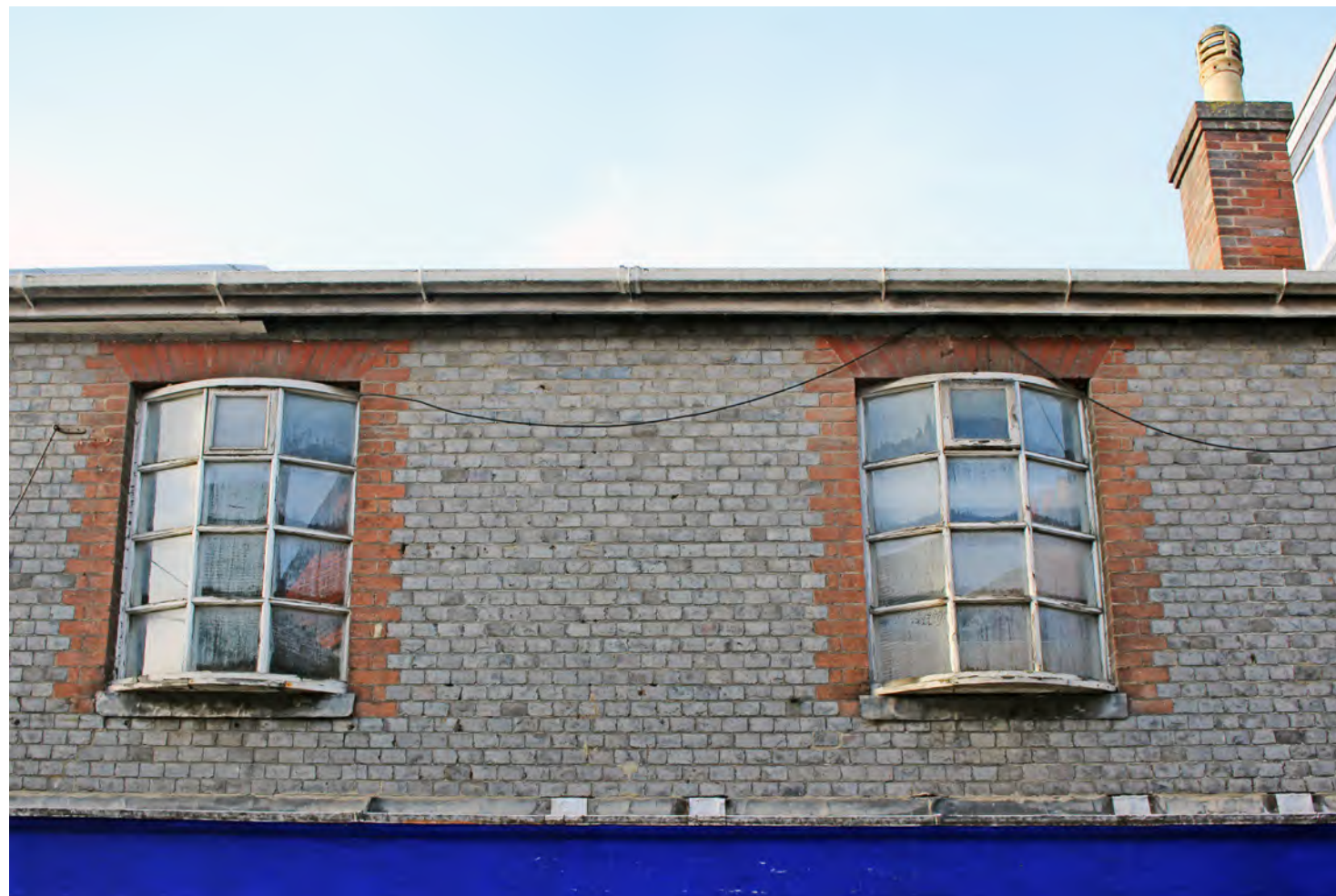
Figure 151: Non-original timber windows in disrepair
