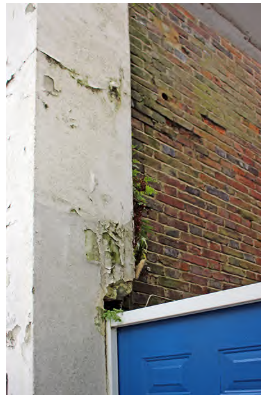
Figure 192: Building fabric in poor repair showing damp and algae due to continued water exposure
