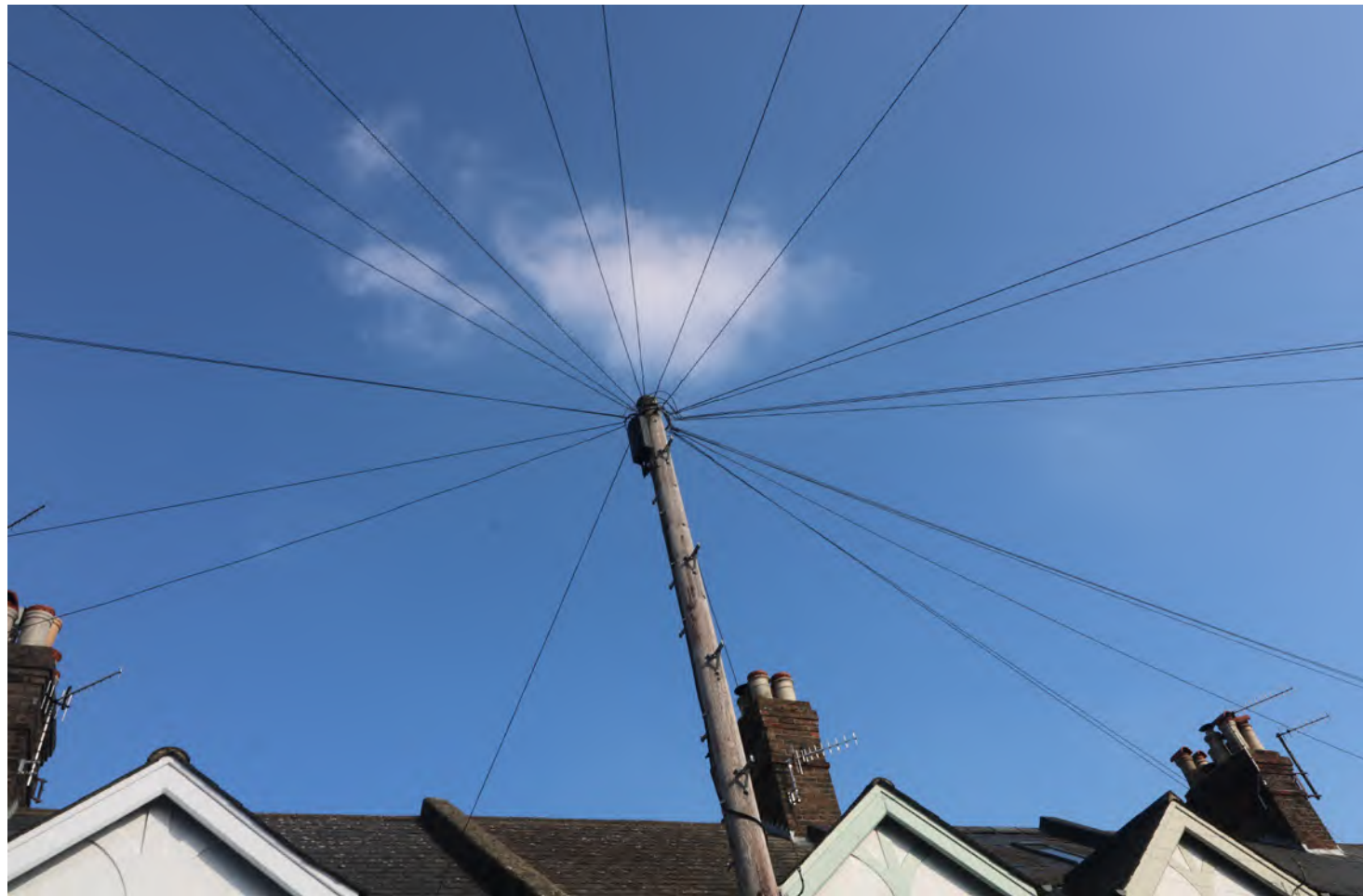
Figure 128: Overhead wires to Morris Road
