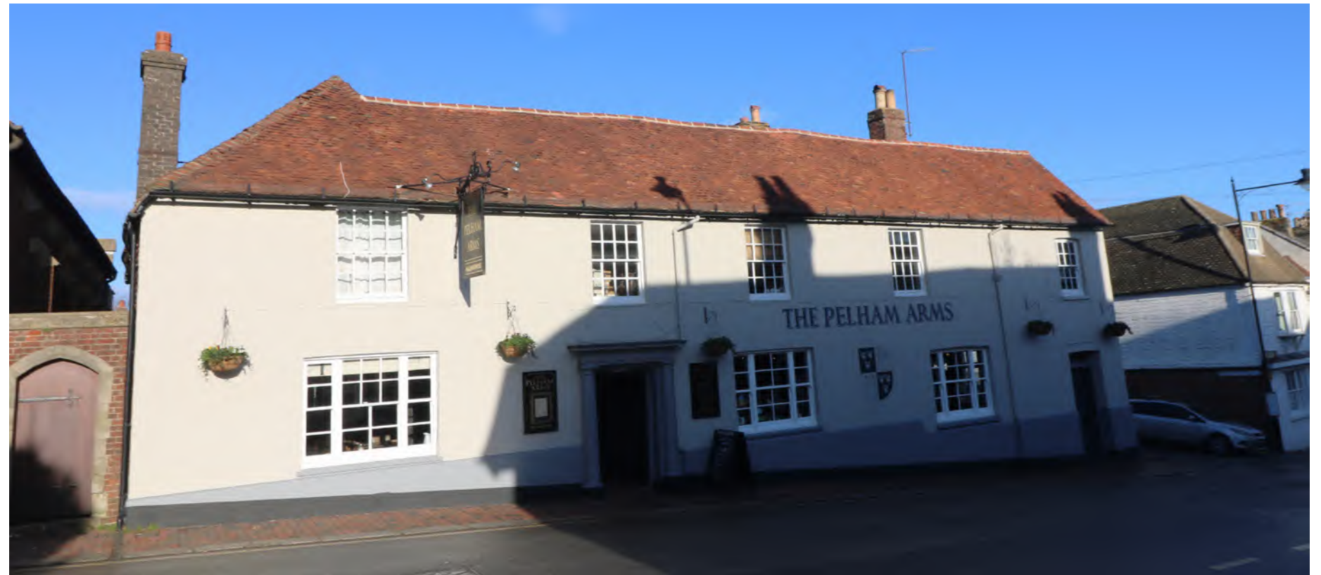
Figure 57: The clay tile roof to The Pelham Arms by St Anne’s Church displays the pleasingly varied shape and colour of handmade clay tiles which makes them such an important part of the Conservation Area’s roofscape
