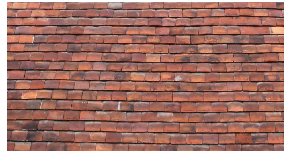
Figure 53: Handmade clay tiles cladding a wall surface . Clear variety in shape, colour and texture
