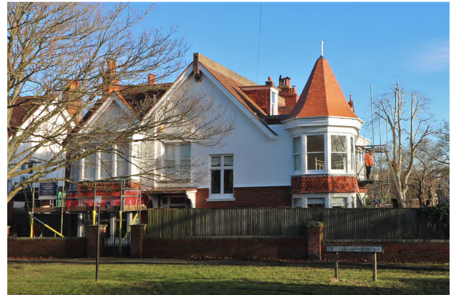
Figure 195: House in the Wallands during repair works, including the sympathetic reroofing of the corner turret
