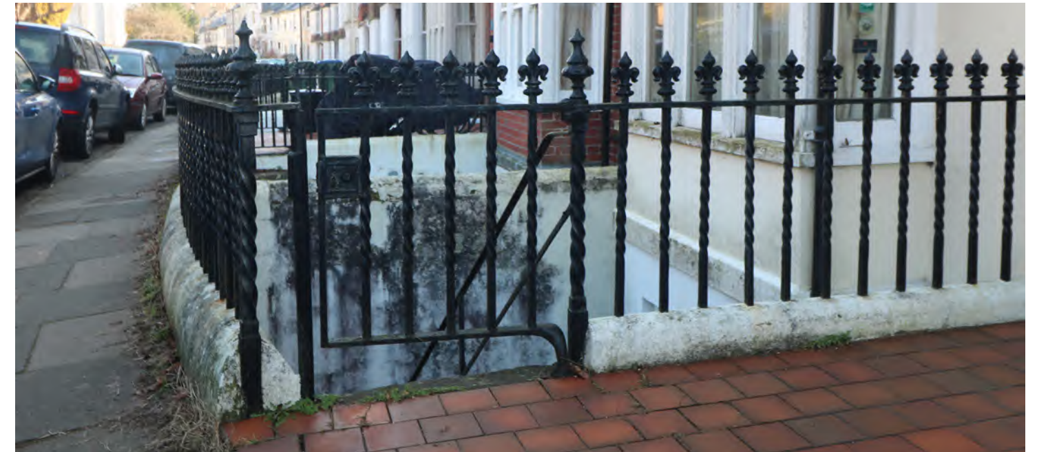
Figure 184: Iron railings to Grange Road
