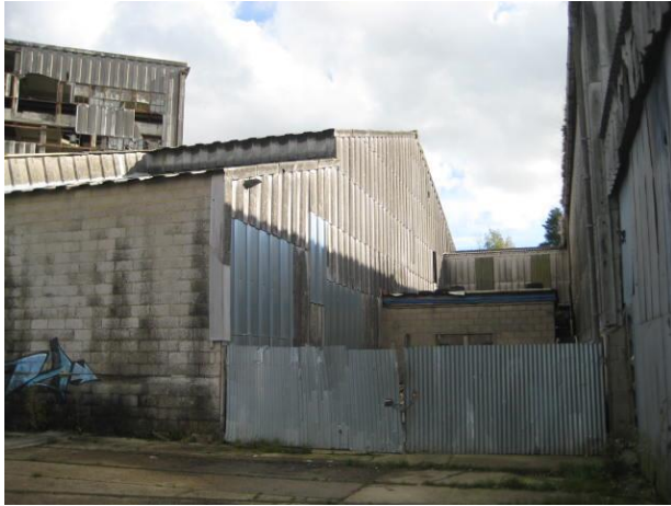
Plate 11: Builders Yard (occupied) – waste materials
