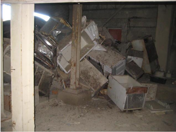
Plate 32: Filter Press house – example of loose corrugated cement sheet
