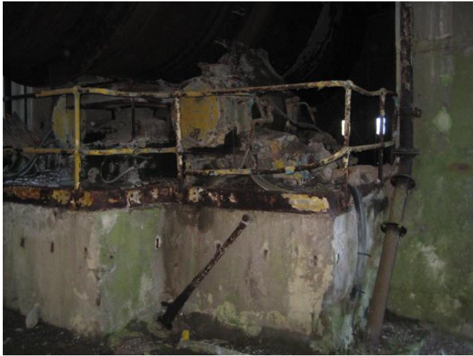
Plate 50: Kiln Shed – flooded pits
