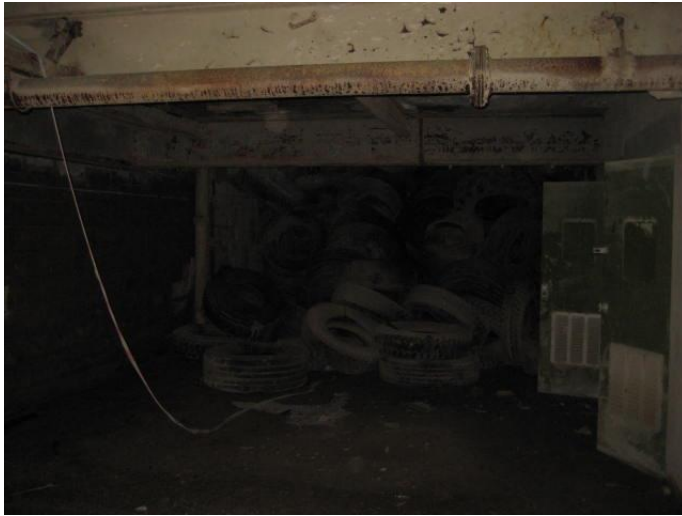
Plate 53: Kiln Shed – side rooms areas in poor condition
