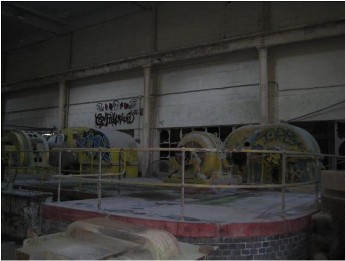
Plate 44: Bunker House – roof in poor condition and breaking-up
