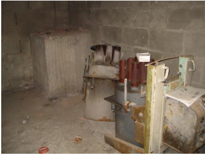
Plate 73: Workshops – discarded electrical switchgear equipment
