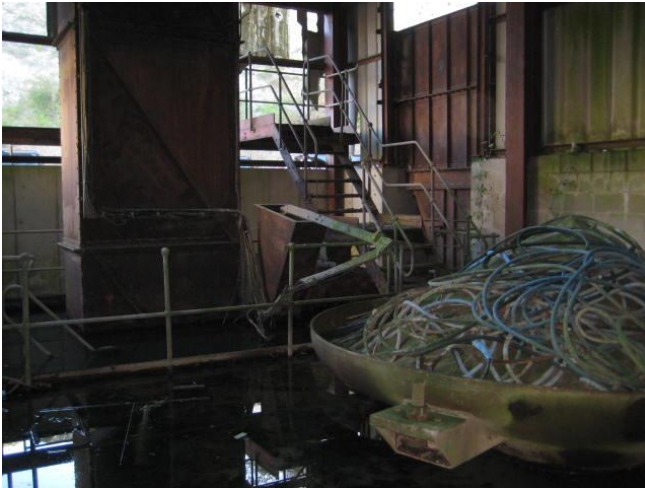
Plate 58: Flooded transfer pit adjacent to Generator House
