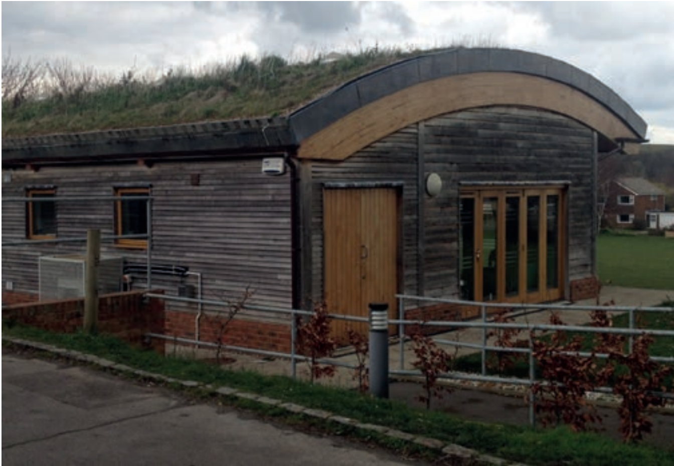
Photo of the green roof on Kingston Village Hall providing insulation for the building, rain water retention and habitat for wildlife. © V Craddock
