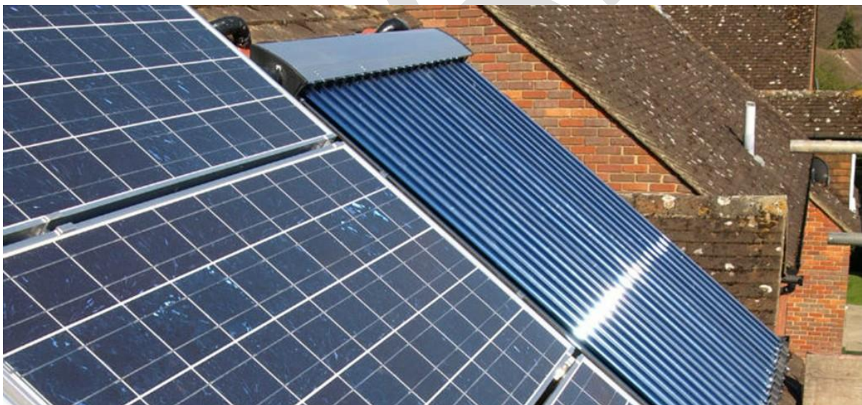
Solar photovoltaic panels (left) and solar thermal panels (right)
