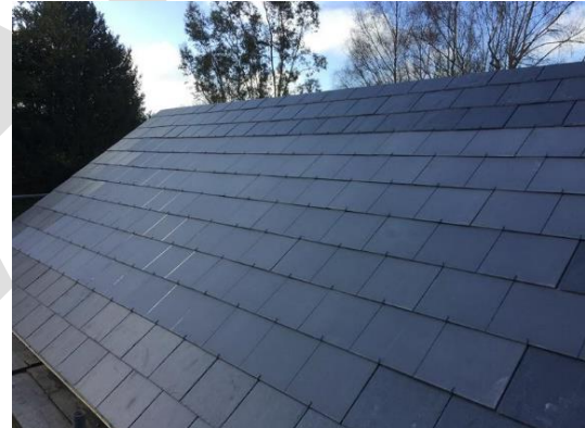
Low visual impact PV tiles on a slate roof
