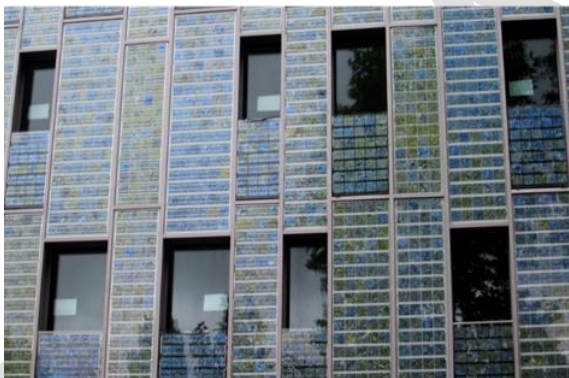
Rain screen cladding PV on an office building
