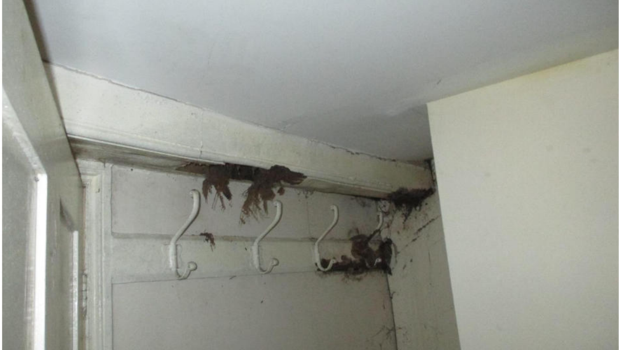
Decayed wall plate
