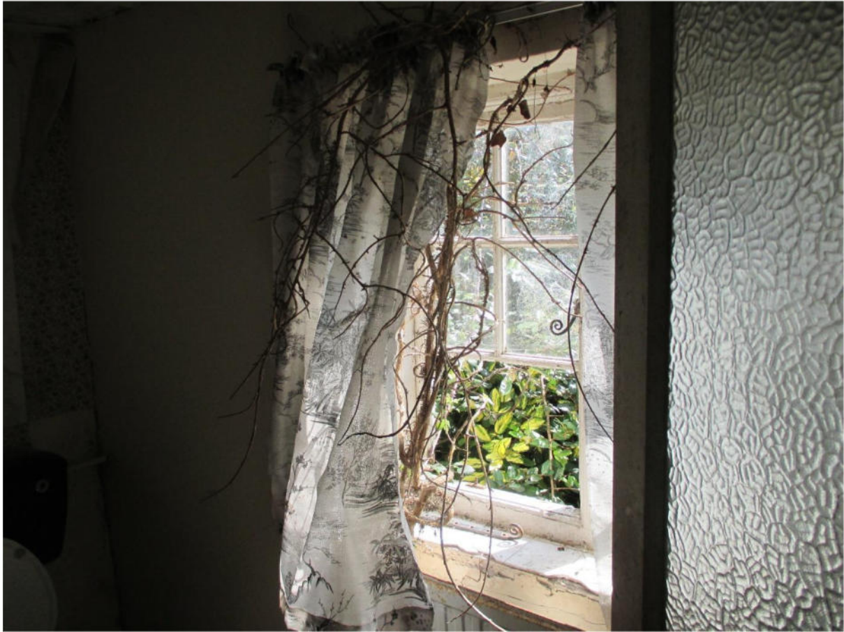
Broken window frame and glazing, seen internally from bathroom
