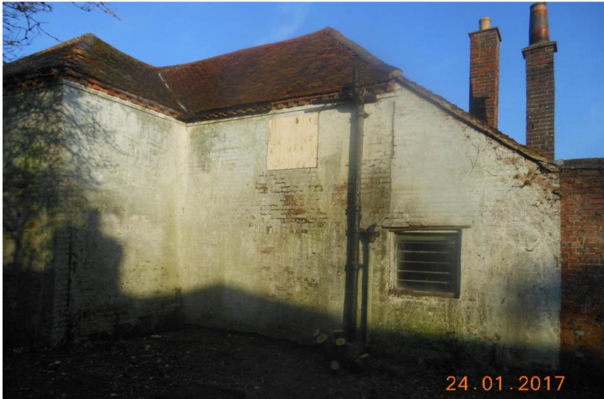
East and South Return faces of Post Office and Cottage to the garden
