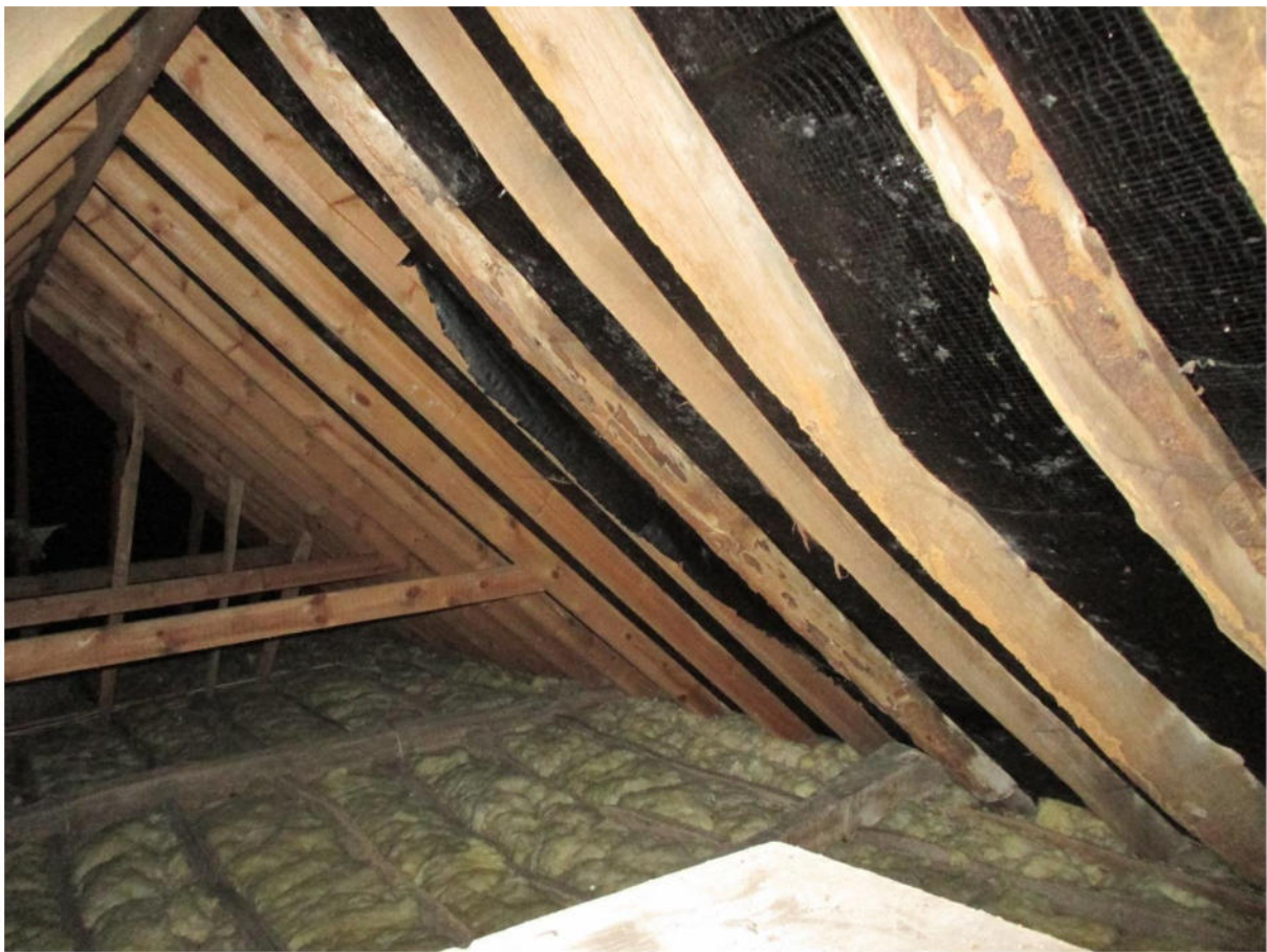
Primary area of over-stressed rafters supporting rear cat slide roof pitch
