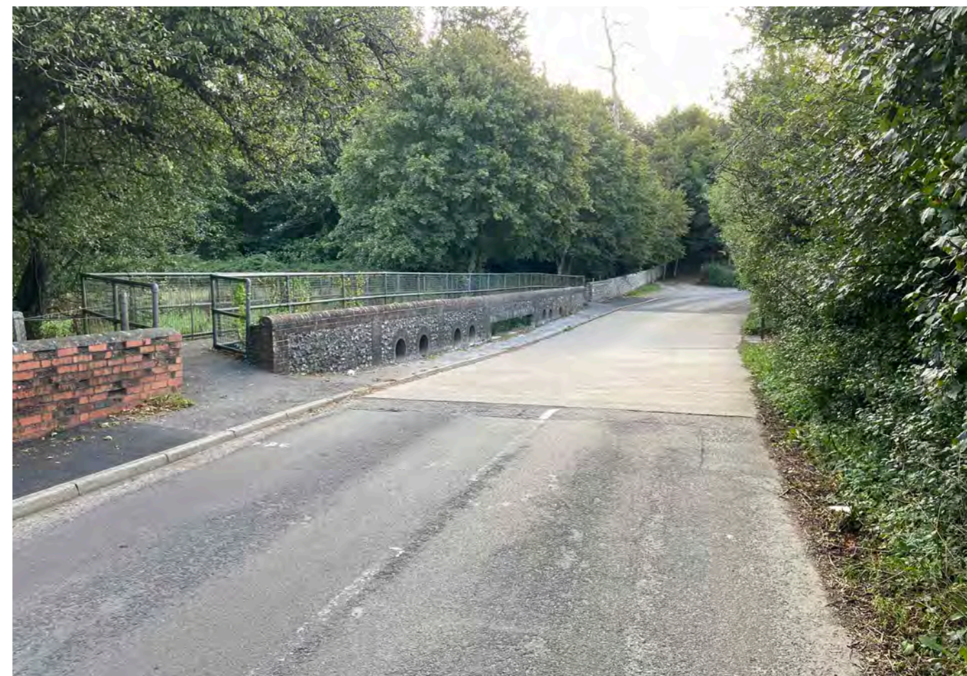
Where the Lavant stream crosses Woodberry Lane traffic movement can be impeded after storm surges
