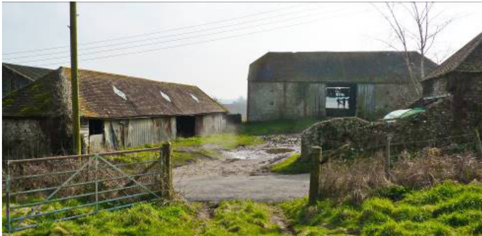
Figure 15: The Southern Farmstead: An 18 th century farmstead which survives intact, along with its farm house (Rock Cottage/Barn Cottage), at the southern end of the settlement.
