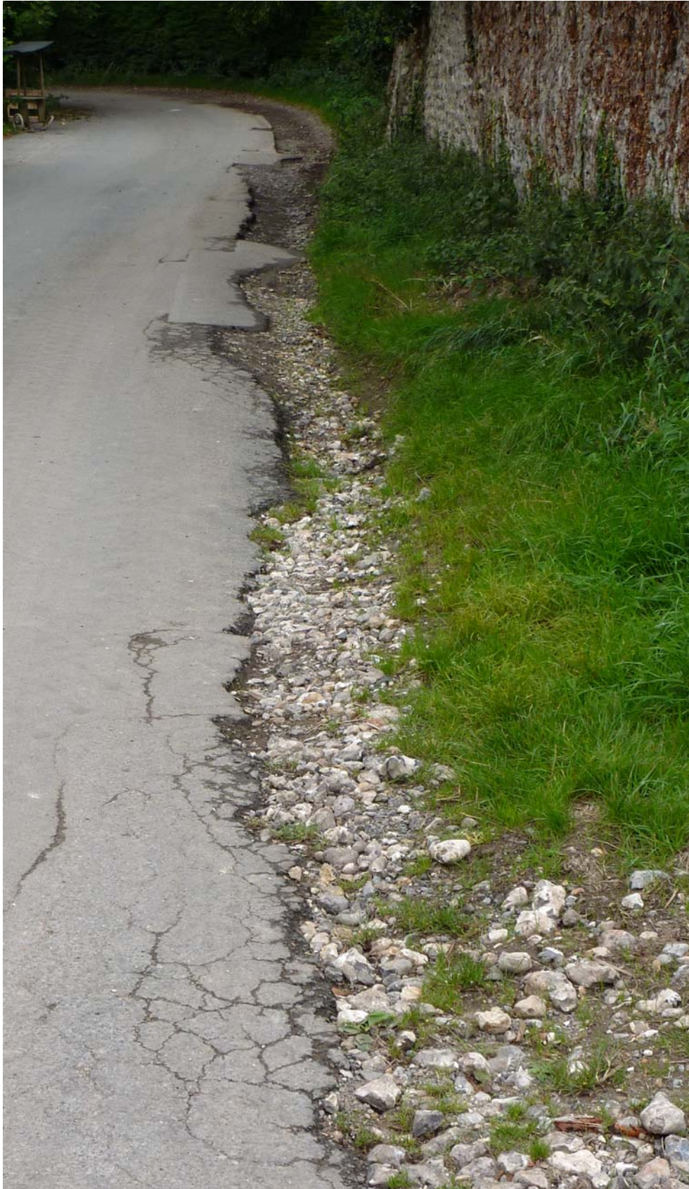
Figure 23: Poor road surfaces on the South Downs Way
