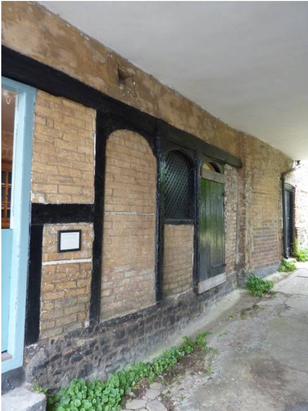
An early screens passage exposed by a later passageway in High Street
