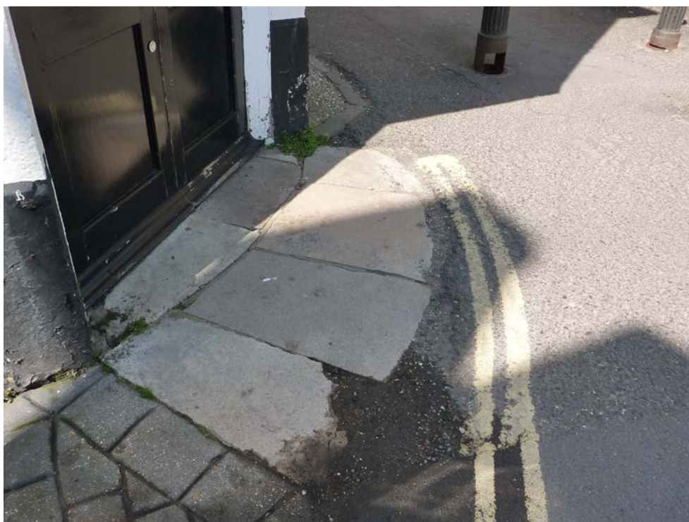
Isolated fragments of historic paving material can still make a local contribution to character and should be retained where possible
