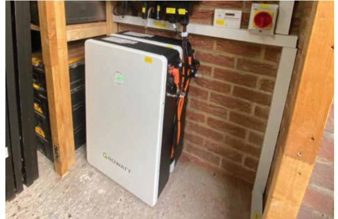
FIGURE 23: A TYPICAL DOMESTIC SCALE BATTERY STORAGE UNIT LINKED TO PV ON A ROOF (SOLARPANELINSTALLERS.UK)
