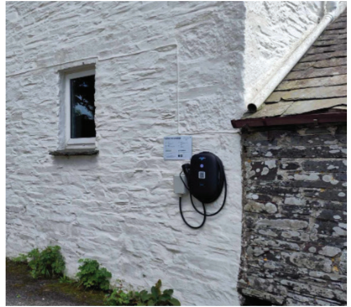
FIGURE 25: A WALL MOUNTED CHARGE POINT (REF: POD ENERGY)
