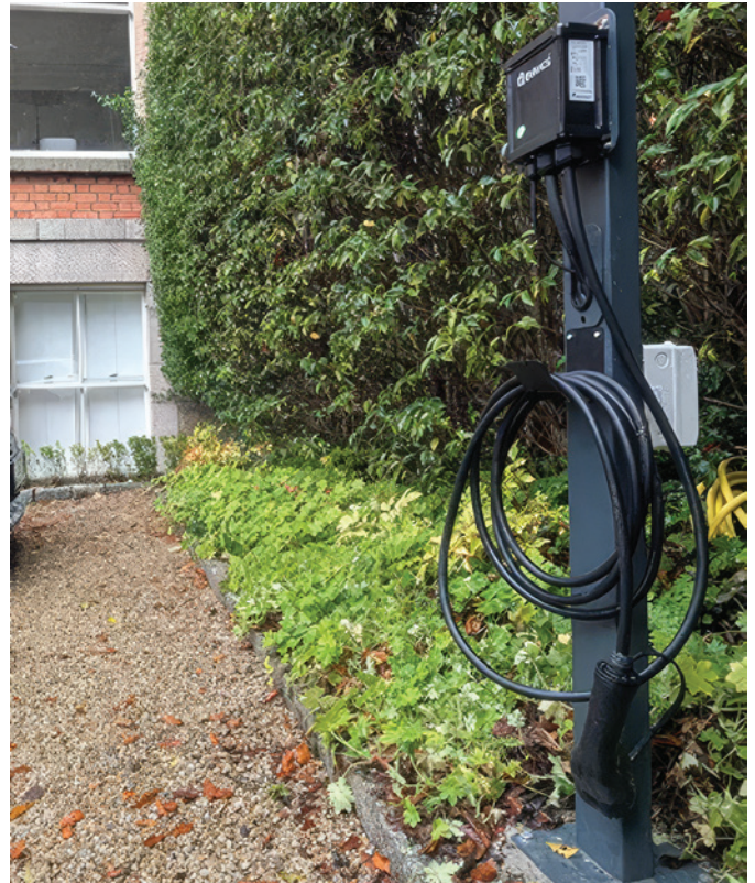
FIGURE 24: FREE STANDING CHARGING POINT IN RESIDENTIAL FRONT GARDEN. (REF: EVHACS)
