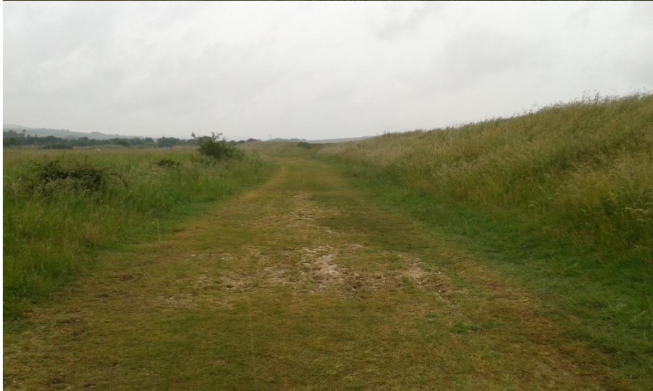
Riverside section below river flood defence (approx Chainage 1350 top and 1250 bottom) looking north, no path and signs of seepage
