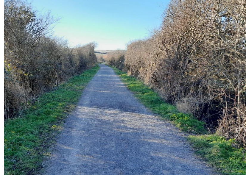
Opened January 2023 NSSC access track - New path constructed 3m width, unbound gravel, limestone dust capped surface
