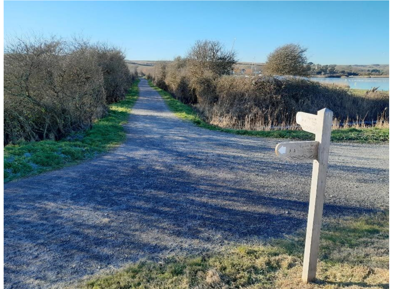
Opened January 2023 NSSC access track - New path constructed 3m width, unbound gravel, limestone dust capped surface
