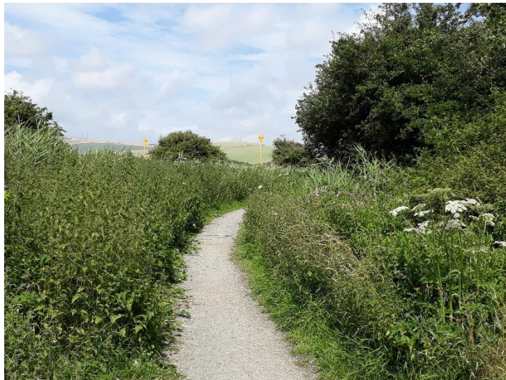
Riverside Park (approx Chainage 1550) looking north Previous degraded gravel surface 1.5m width, narrowing to <0.8m
