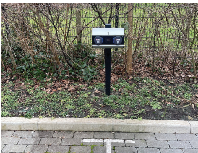
FIGURE 21: FREE STANDING DOUBLE CHARGE POINT IN RESIDENTIAL CAR PARK, MIDHURST
