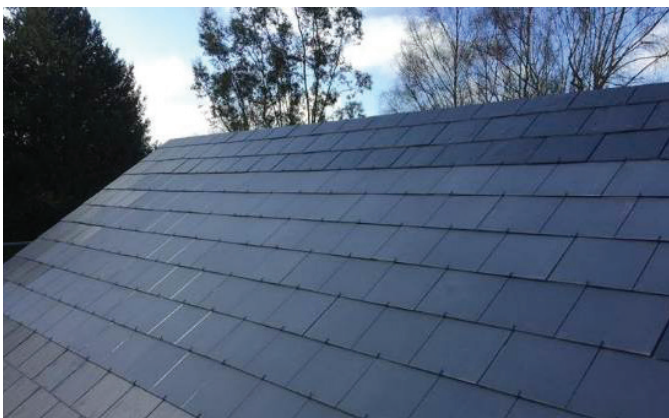
FIGURE 13: LOW VISUAL IMPACT PV TILES ON A SLATE ROOF
