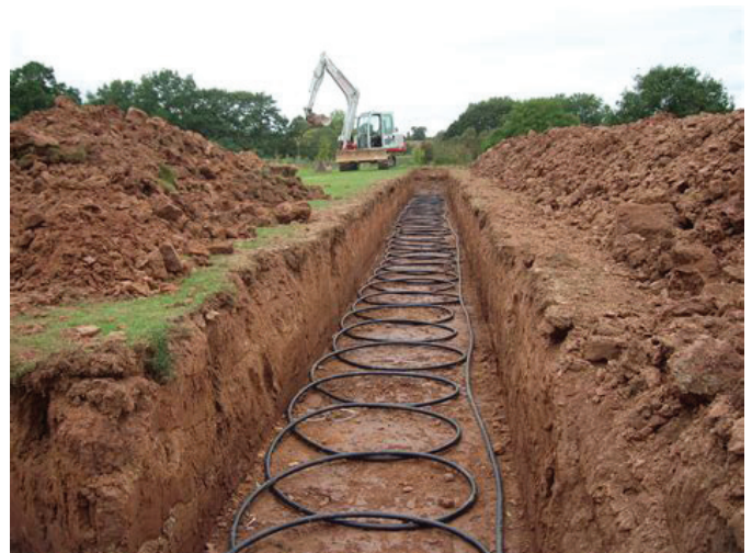
FIGURE 18: TYPICAL EXCAVATION AND INSTALLATION OF VERTICAL GROUND SOURCE HEAT PUMP LOOP (SELF BUILD)
