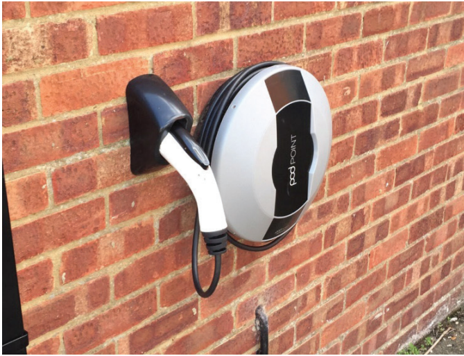
FIGURE 22: A WALL MOUNTED CHARGE POINT
