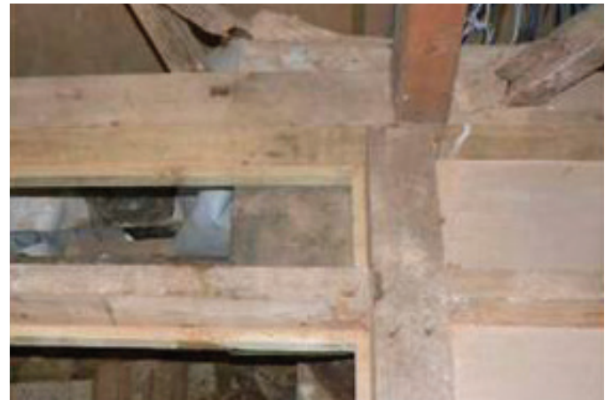
FIGURE 4: BATTENS ADDED AT THE SIDES OF THE JOISTS TO SUPPORT BOARDING & CARRY COMPRESSIBLE SHEEP'S WOOL INSULATION IN A SUSPENDED FLOOR
