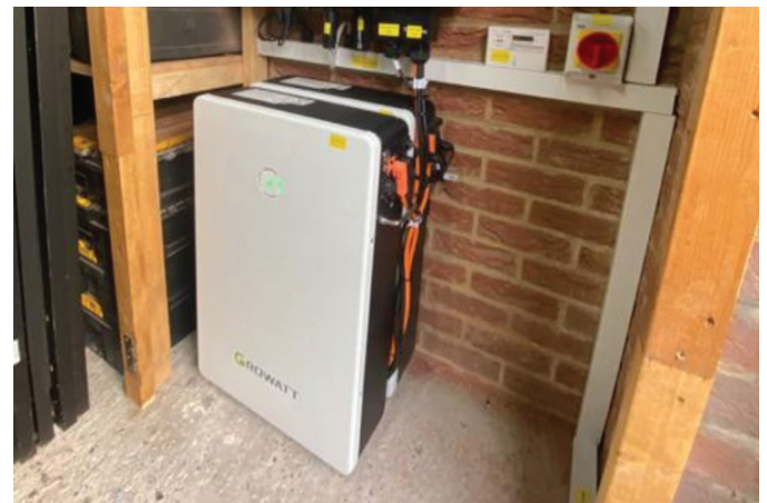
FIGURE 20: A TYPICAL DOMESTIC SCALE BATTERY STORAGE UNIT LINKED TO PV ON A ROOF (SOLARPANELINSTALLERS.UK)
