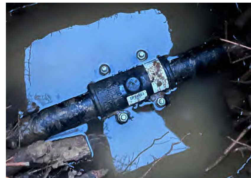
A fixed joint following a leak in 2024
