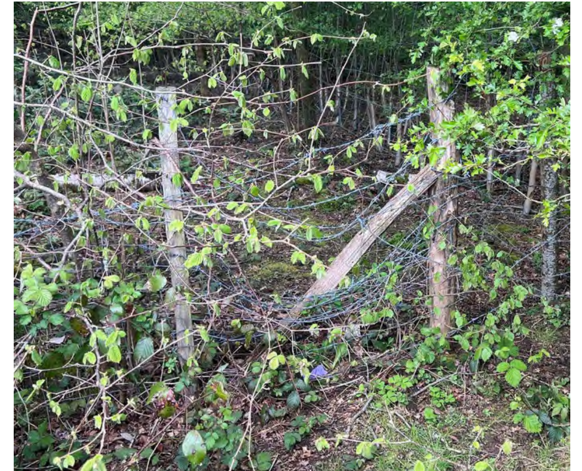
One of many fences at Foley that needs replacing
