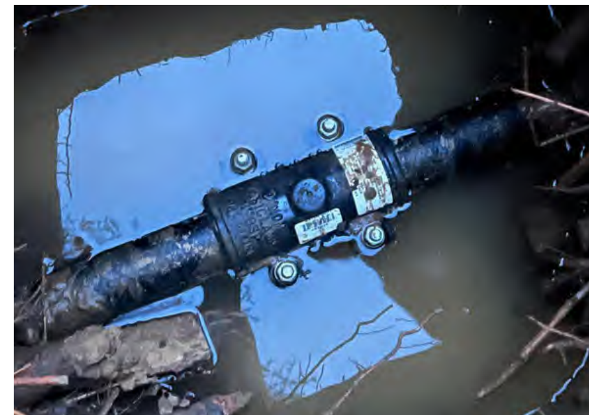
A fixed joint following a leak in 2024
